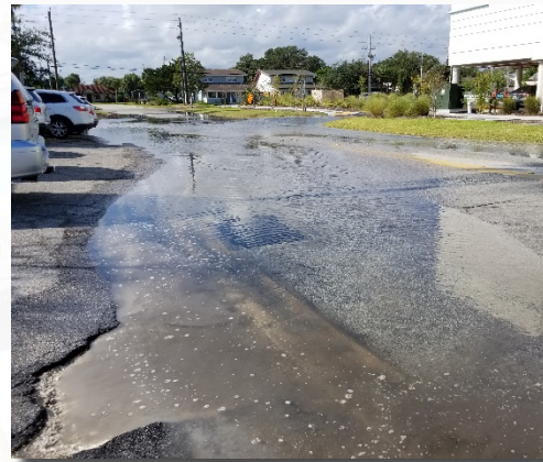
Nuisance flooding prior to one-way tidal valve installation
